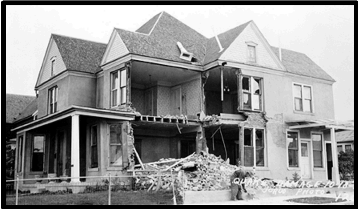
This residence at 1601 Lyndale Avenue, Helena, Montana, illustrates the typical partial failure of a brick bearing-wall dwelling. Photo by L.H. Jorud, Helena, MT; from MT Historical Society collection.
