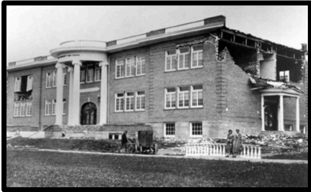
Brick wall and parapet fell from new Community High School in Manhattan, Montana. Photo by J.T. Pardee
