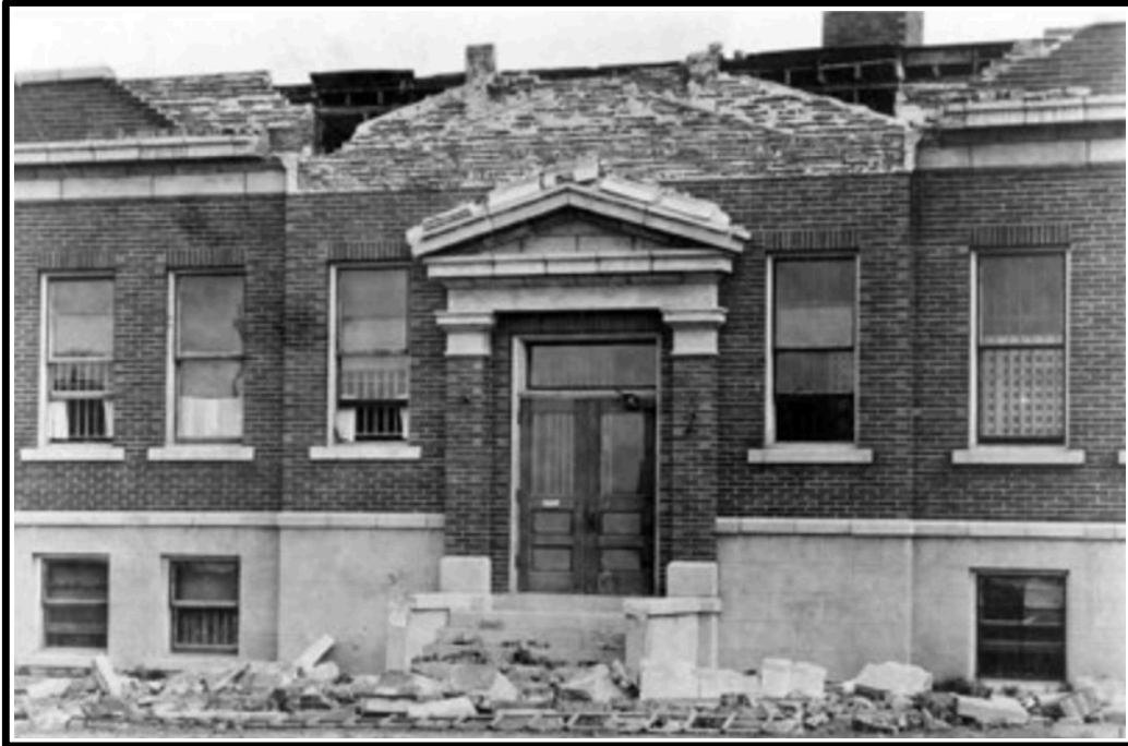
Brick veneer sheered from back wall of jail in White Sulphur Springs, Montana. Photo by J.T. Pardee.
